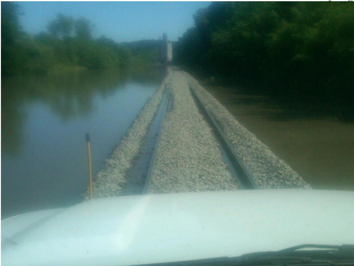
Falls City Sub
