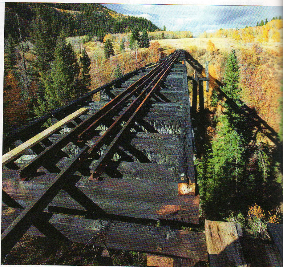
The Lobato Trestle, constructed in 1883, was damaged but not destroyed by fire last year. Engineers determined that those elements untouched by the fire remained in good condition.
